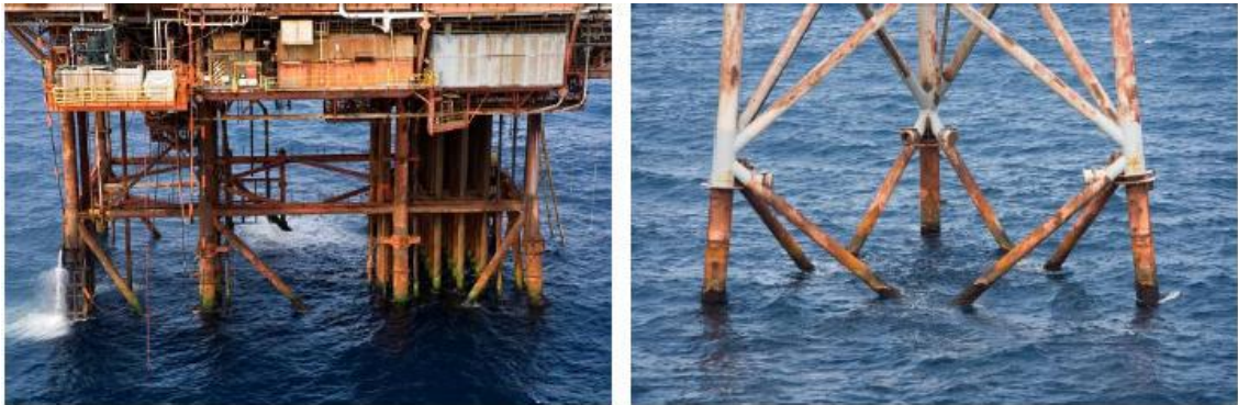
Figure 1 and 2: Pictures of Platforms.
