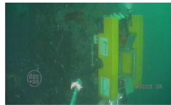
Above image is from the ROV during the inspection of Leg K3.
