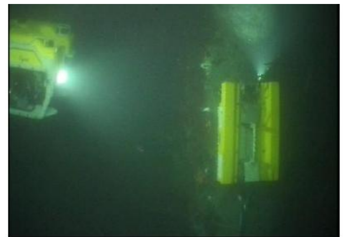
Above image is from the ROV during the inspection of Leg K2.
