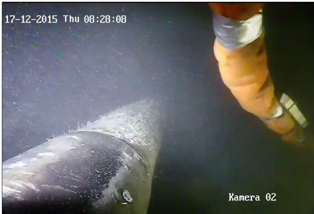
Figure 4: Camera View on Section A of XXXX pipeline
