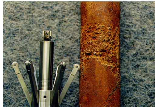
External corrosion near the lower bend
