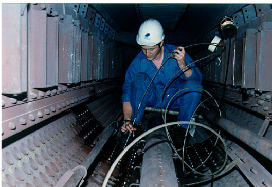
Inspection of steam drum. Tubes are plugged from the mud drum and filled with water
