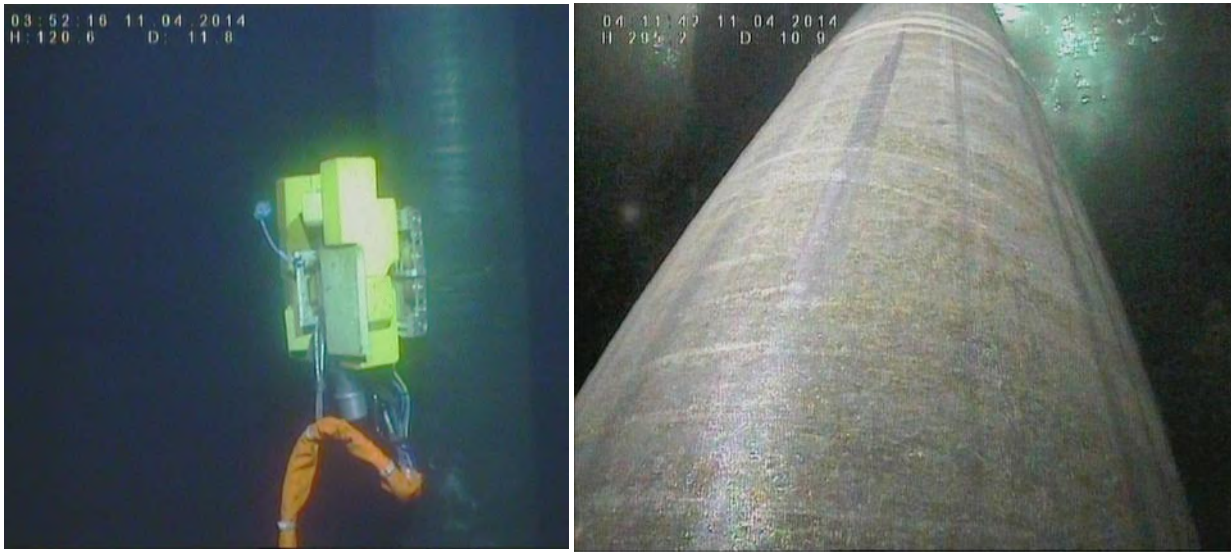
Figure 6: Video screenshots of MEC-Combi crawler inspecting caisson xx (left) and view from the front camera of the tool (right)
