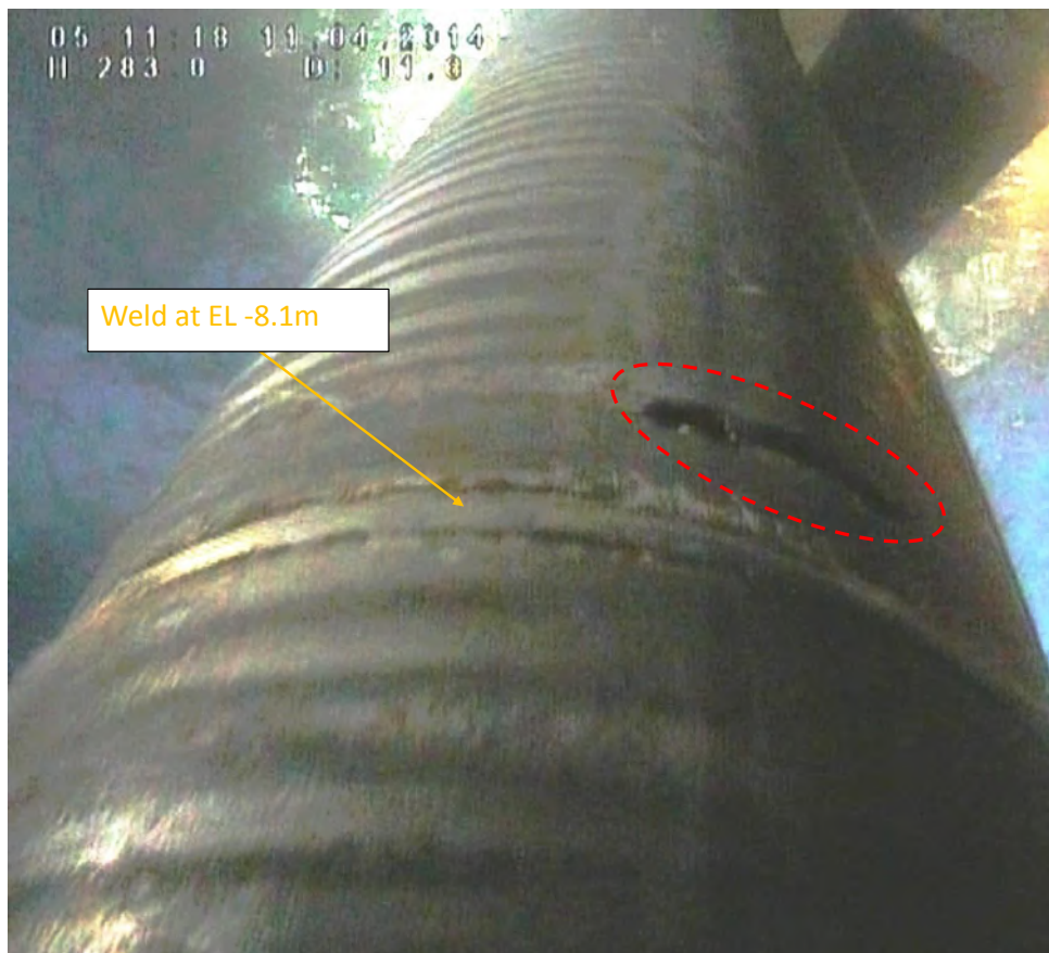
Figure 11: View of the south-western weld region of xx at EL -8.1 m (screenshot from video file of Track 14). The area marked in red corresponds to the external indications shown in Figure 9.
